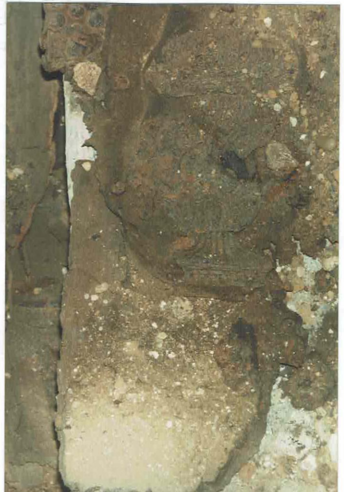
A CORRODED CREST
