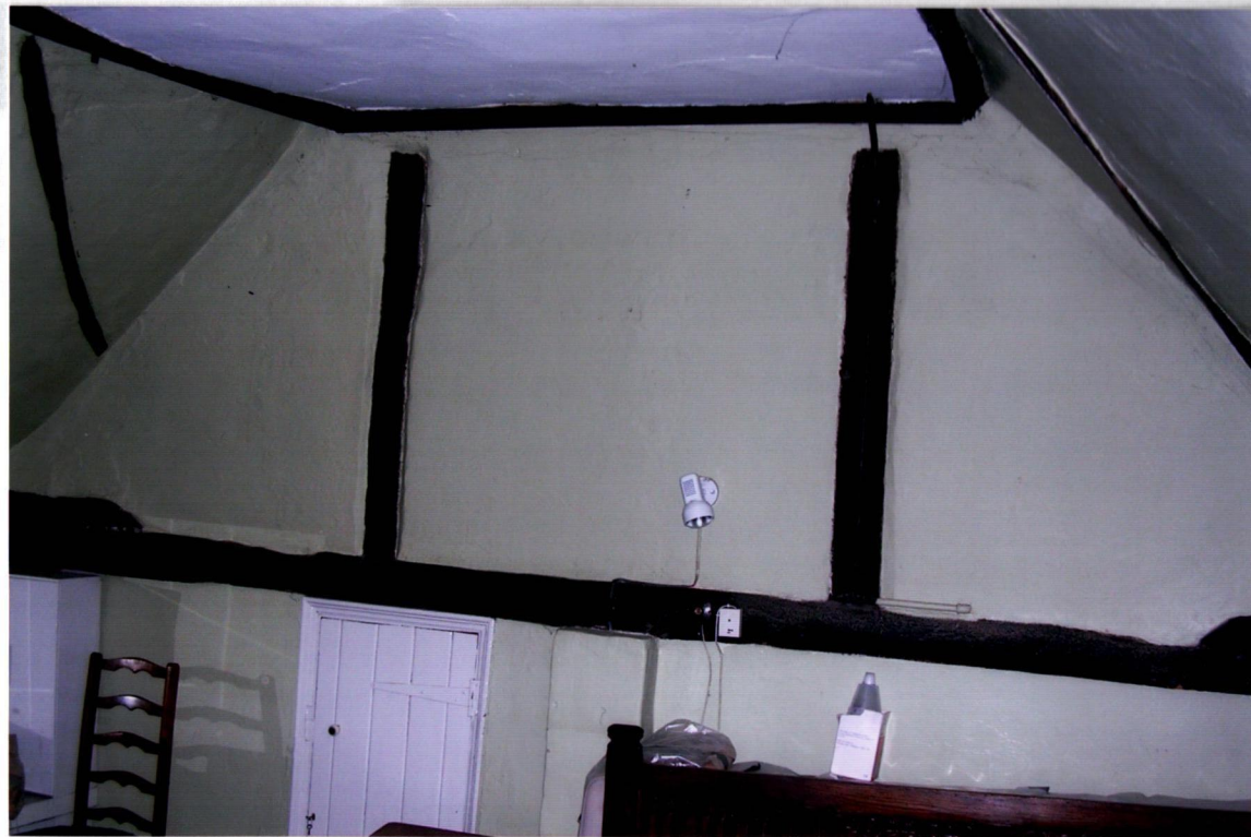
1 st floor of hall looking SE Queen posts and tie beam replace originals, however, ends of tie beams are visible on extreme left and right
