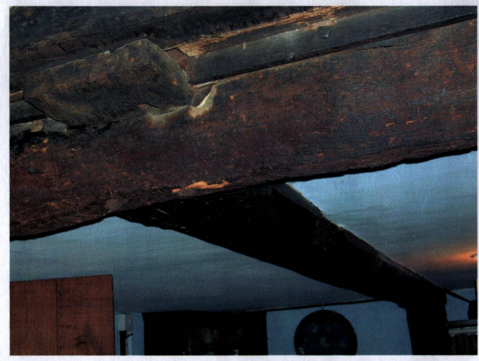
Crosswing: transverse beam, SE end tenoned through bressumer. Chamfer and charring on bressumer suggest former hearth use.
