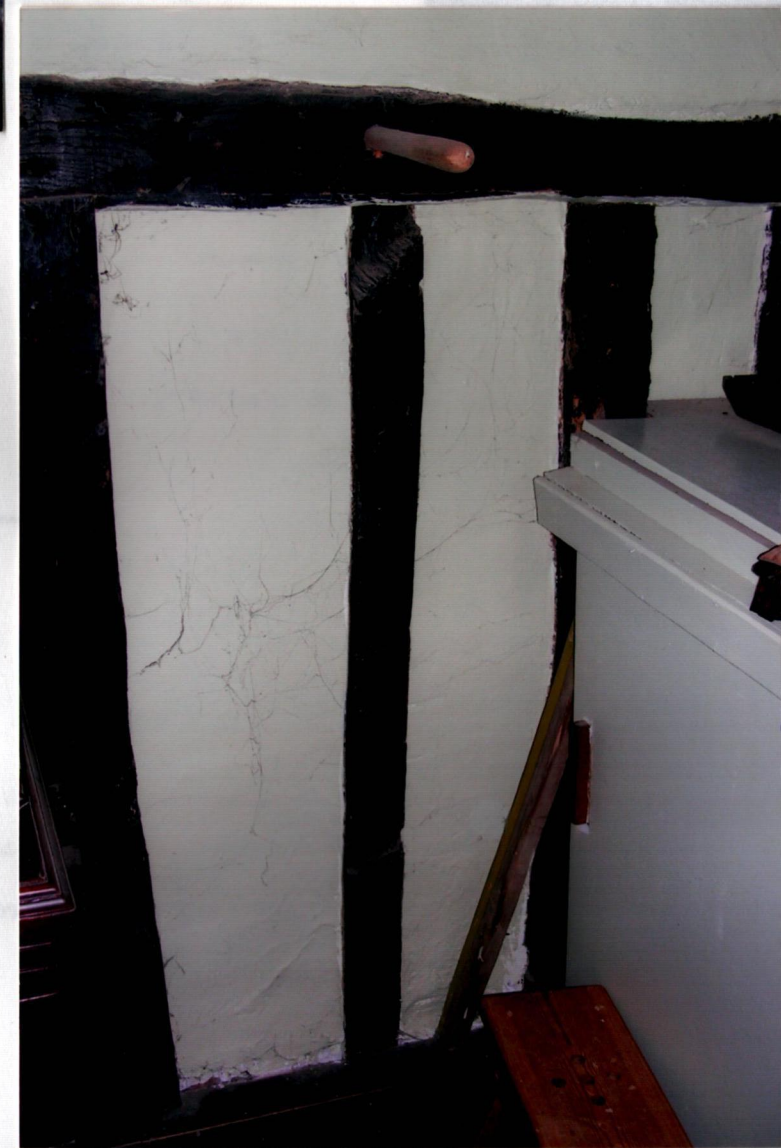
1 st floor of hall, N.W. end Riven struts mark like of smoke bay, backing onto crossing
