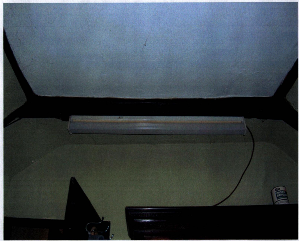
1st floor hall, NW end. Collar (with attached strip light) has stove holes to underside, indicating former panel for smoke bay.
