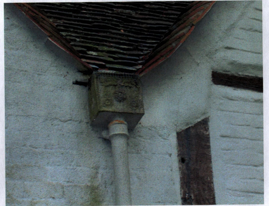
Exterior: NE side: Detail of rainwater hopper at the junction of the gables.
