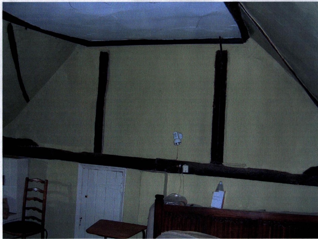
1st floor of hall looking SE. Queen-posts & tie-beam replace originals, however, ends of tie-beams are visible on extreme left & right.
