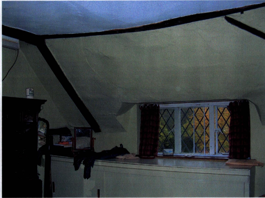
1st floor of hall looking NE. The rafter and collar to the left, mark the line of the probable smoke-bay. Note wind brace top right (visible in photo below on the left).
