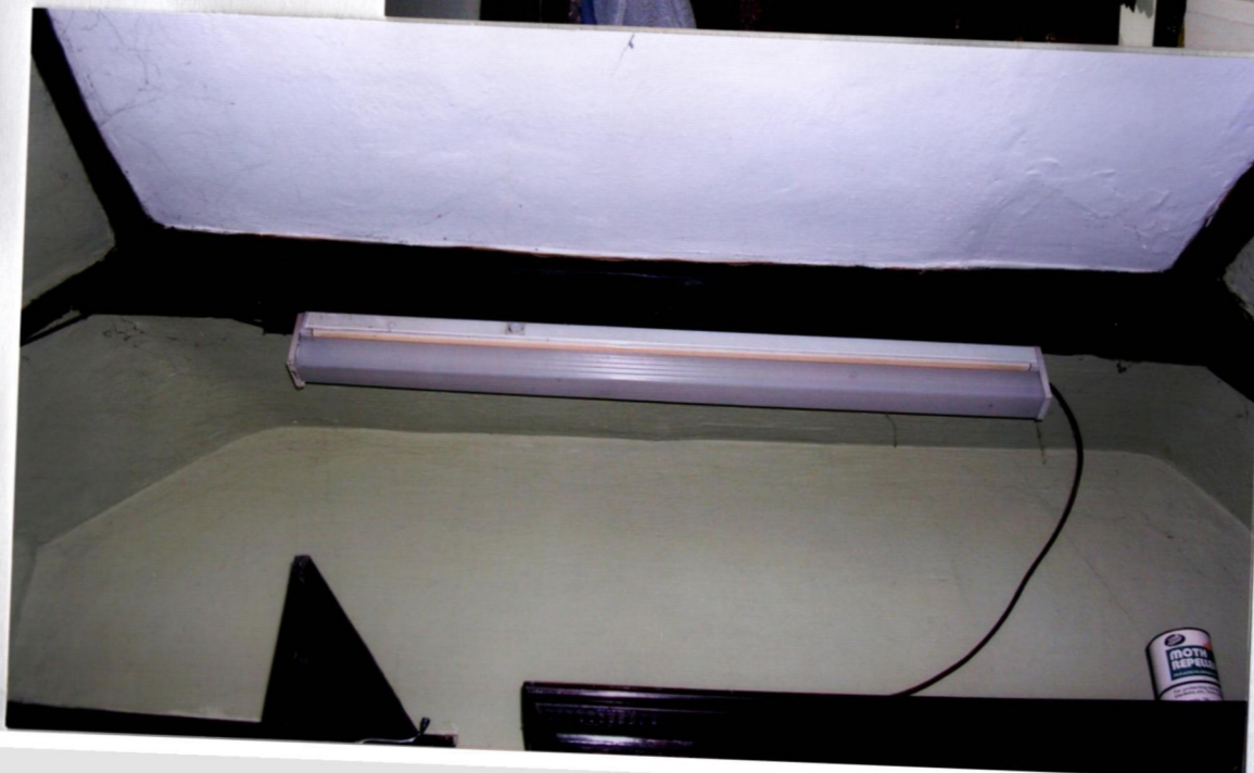
1st floor hall NW end collar (with attached strip light) have saw holes to underside, indicating former panel of smoke bay
